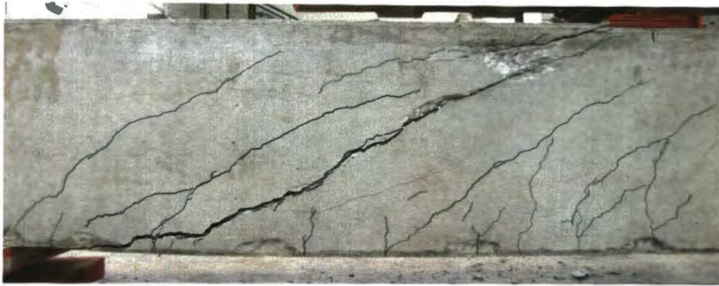
Figure 6.49. Control-5-1 Beam at Failure
